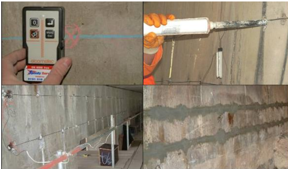
Figure 4 Stages in a hybrid treatment process showing (a) locating the steel, (b) installing the anode system (c) the impressed current treatment and (d) the galvanic protection phase.
