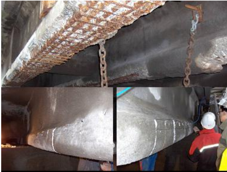
Figure 11 Reinforced concrete beams in a marine structure prior to (top) and after repair and treatment (bottom left and right).
